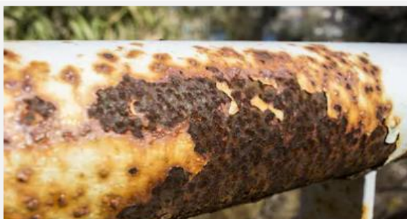
EXTERNAL CORROSION (REINFORCEMENT)
