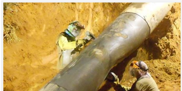
MECHANICAL DAMAGES (REINFORCEMENT)
