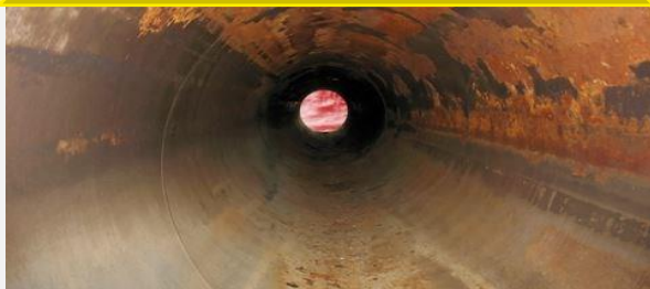
INTERNAL CORROSION (REINFORCEMENT)
