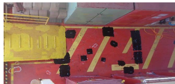
Fig. 7: Deck overview with several patching repairs
