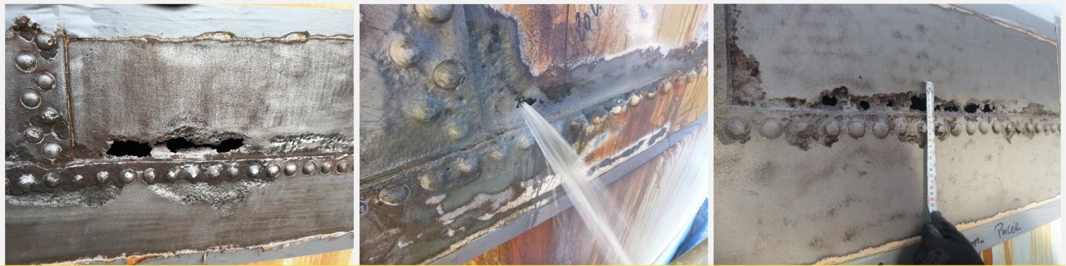
EXAMPLES OF DEFECTS TO BE REPAIRED – BEFORE REINFORCEKIT® PATCH
