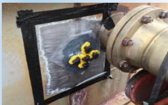
Fig. 4: Metallic plate application over the defect using magnets
