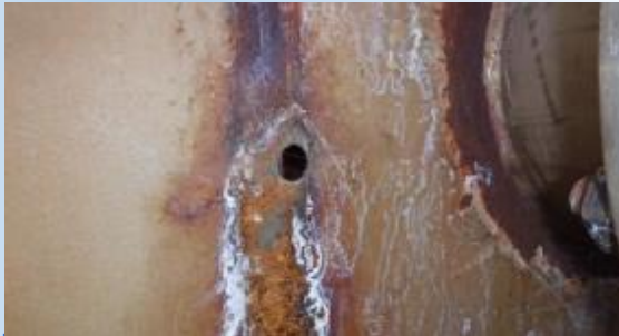
Fig. 1: View of the defect
