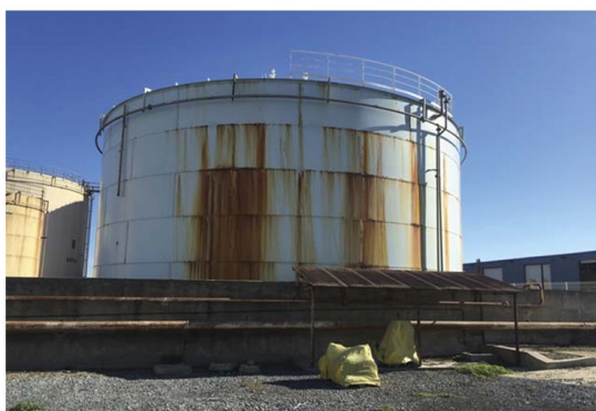
Figure 1. General view of corroded water tank before REINFORCEKIT® PATCH installation.
